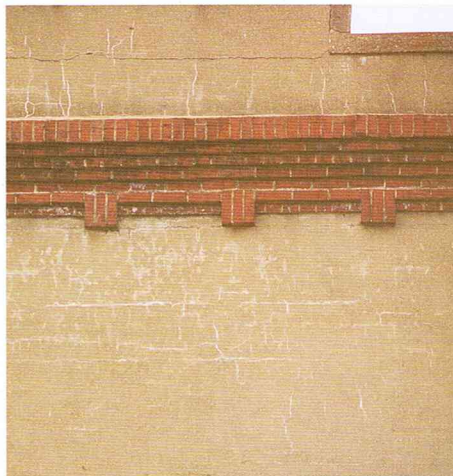
Fig. 4 Plaster wall cracked and discolored after a while in the open.
